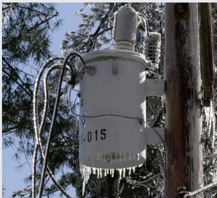
Ice accumulations exceeded .6 inches in some areas of Ulster County.
