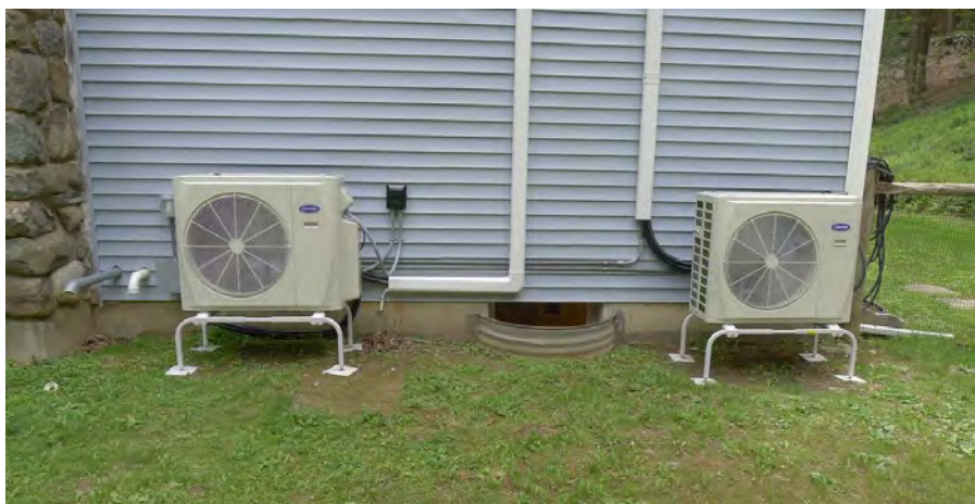
Figure 23: Air Source Heat Pump System Installed at a Central Hudson Customer Residence
